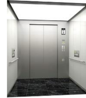
Elevator Floor Control
